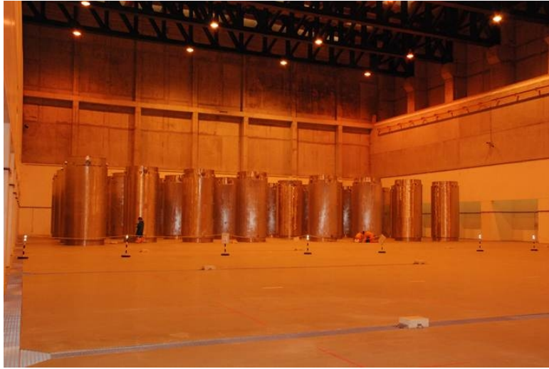
The interior of the ITS at the Trillo nuclear power plant.
